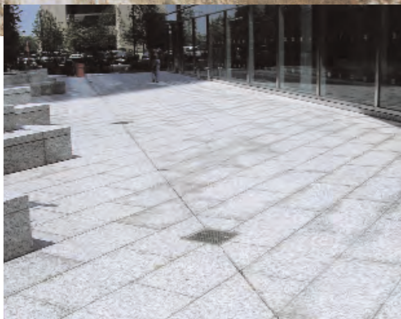
Moisture damage on exterior floor slabs.
